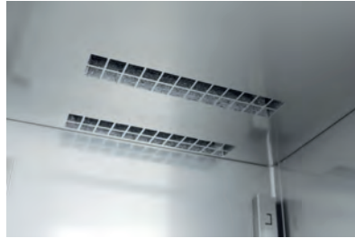
Detail of internal ventilation
