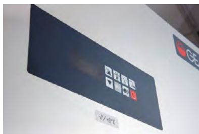
Back panel control board
